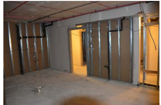
Picture 2 - Banquet Kitchen
