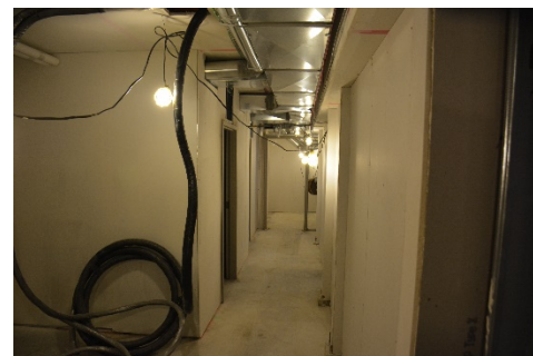
Figure 5- Mechanical Room Hallway (also to Cadet Office)
